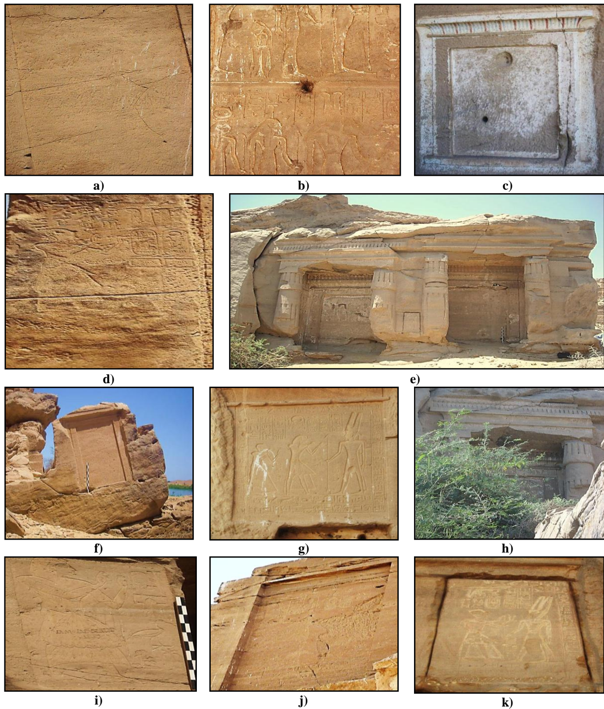
Figure 2. Deterioration aspects of rock-cut panels at Gebel el-Silsila: a) Fissures and cracks; b) Loss of white wash; c) Loss of mortar; d) Discoloration and rising moisture; e) Erosion by the water of the Nile during flood and fractures in rock cliff; f) The inclination and the subsidence; g) Soiling by bird droppings; h) The vascular plants; i) Visitor's scribbles by scratching; j) Removing the inscriptions; k) Looting and cut for selling.
