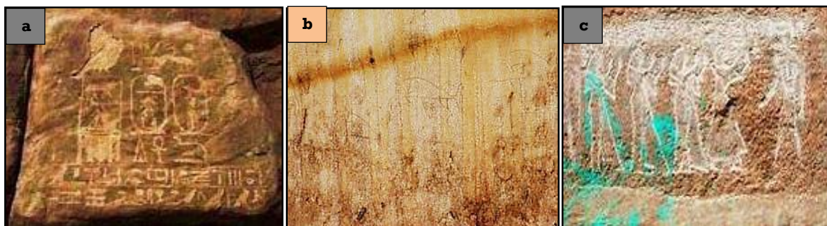
Figure 3. Deterioration phenomena of studied rock art: a) exfoliation; b) discoloration due to rains and inappropriate treatment; c) aesthetic disfigurement due to synthetic paints and chalk.
