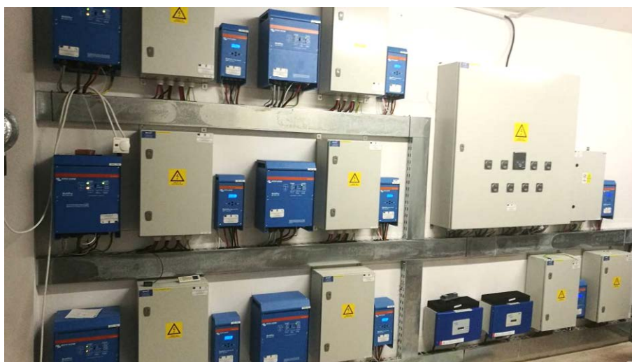
Figure 4. Microgrid power distribution room.
