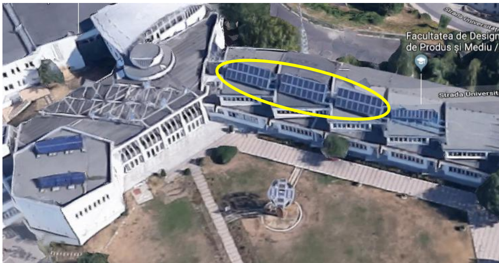
Figure 1. On-grid 9.6 kWp photovoltaic system installed on the Colina Hill rooftop facilities of the Renewable Energy Systems and Recycling R&D Centre, Transilvania University of Brasov.
