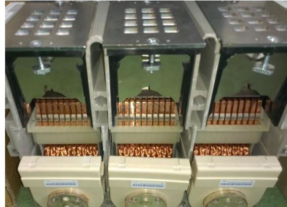
Figure 13. The Low Voltage Circuit Breakers.
